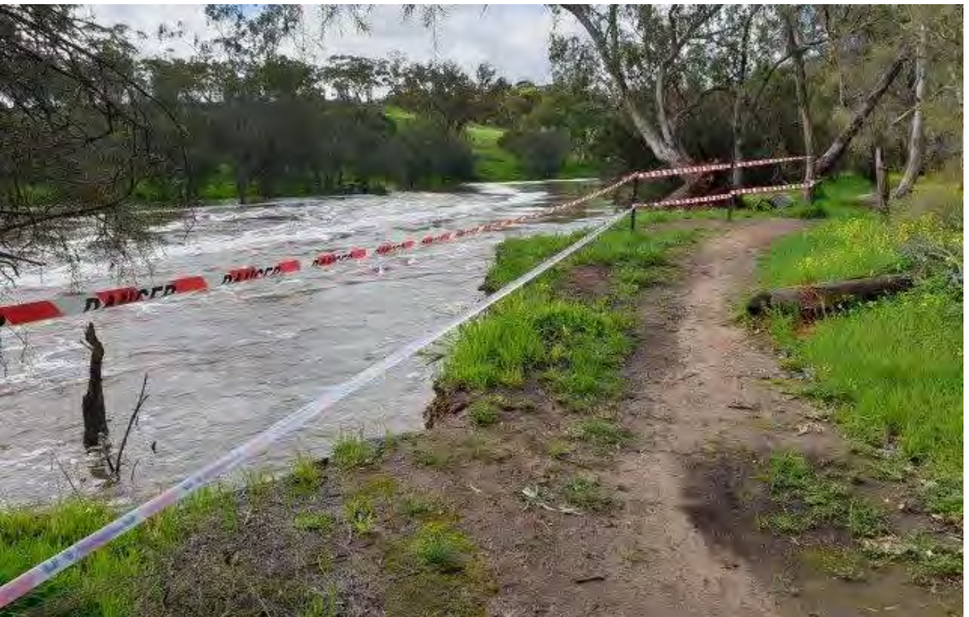
Above: Collapsed bank next to the Bilya Walk Track
